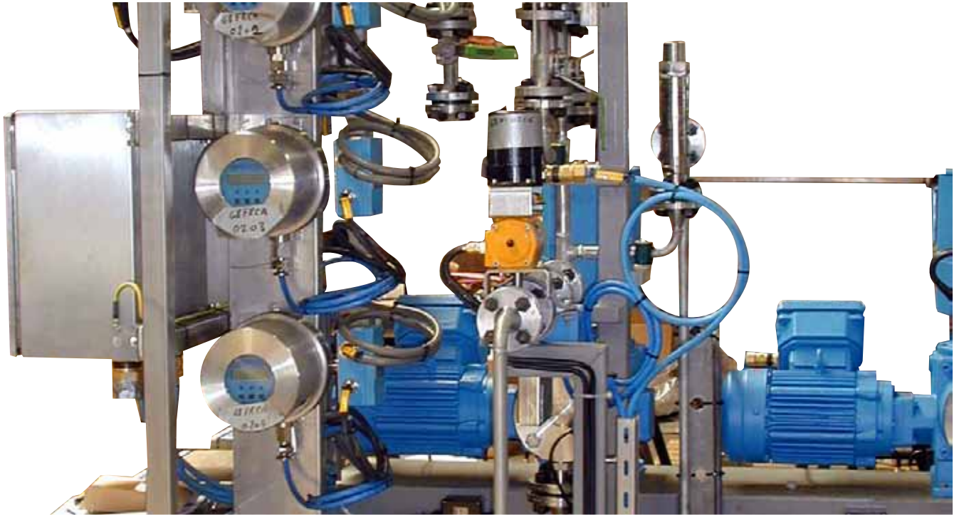
Oil & gas flow metering skid
